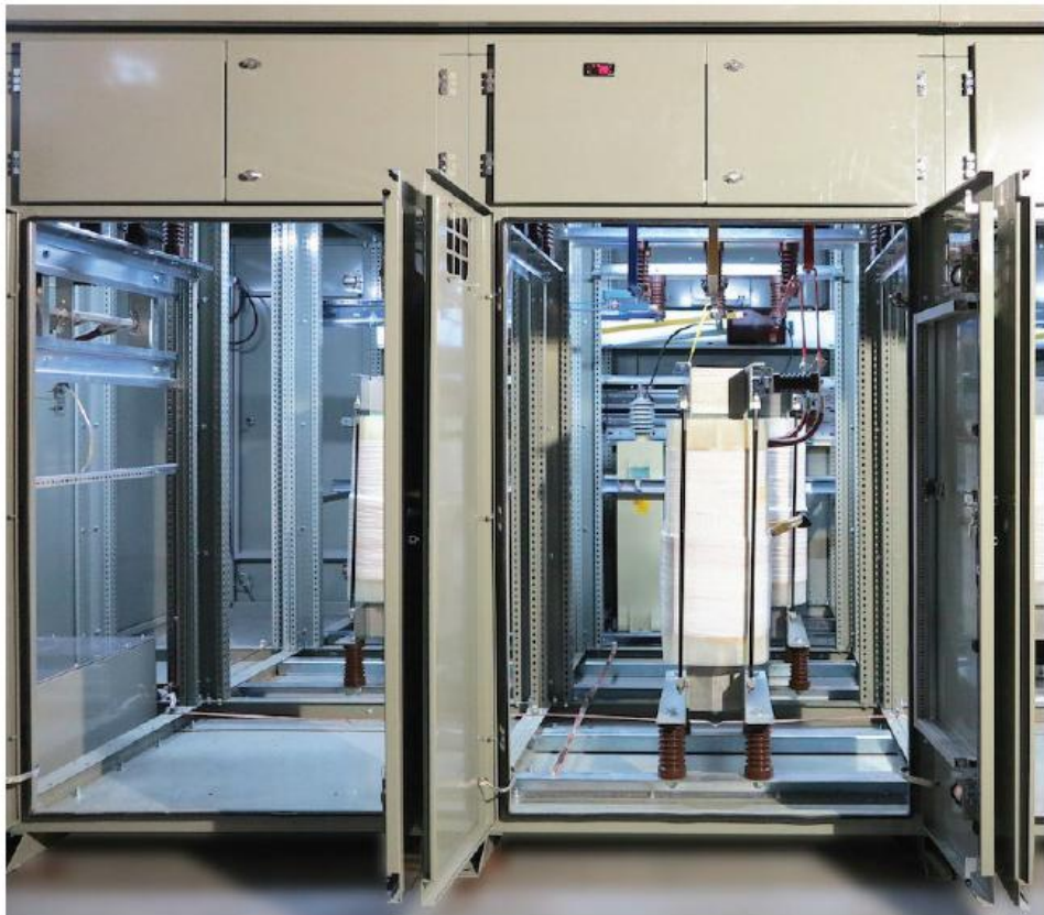
33kV Outdoor Bank with Detuned Reactors IP54 RAL7035 Painted Panel
